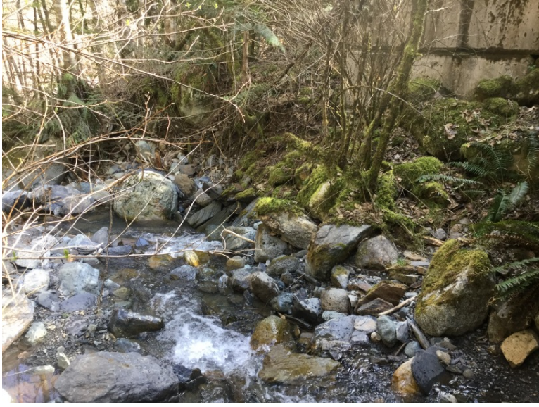
Downstream right abutment scour
